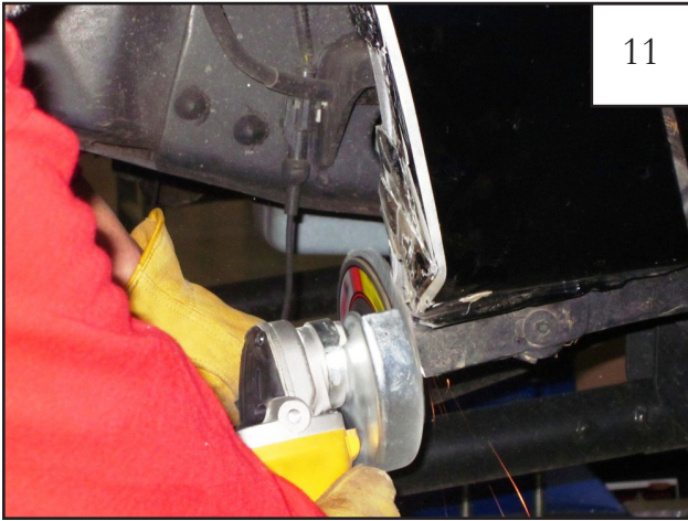
Using a hammer and an angle grinder, flatten tabs then grind down any sharp edges. Treat any bare sheet metal with rust resistant paint BEFORE continuing.
