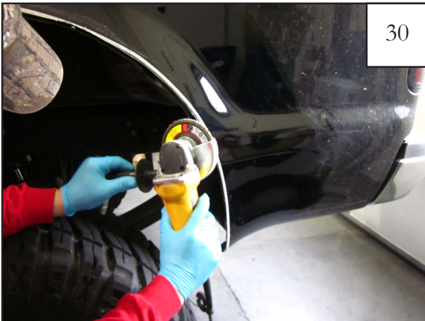
Using a grinder, debur cut edges. Treat any bare sheet metal with rust resistant paint BEFORE continuing.
